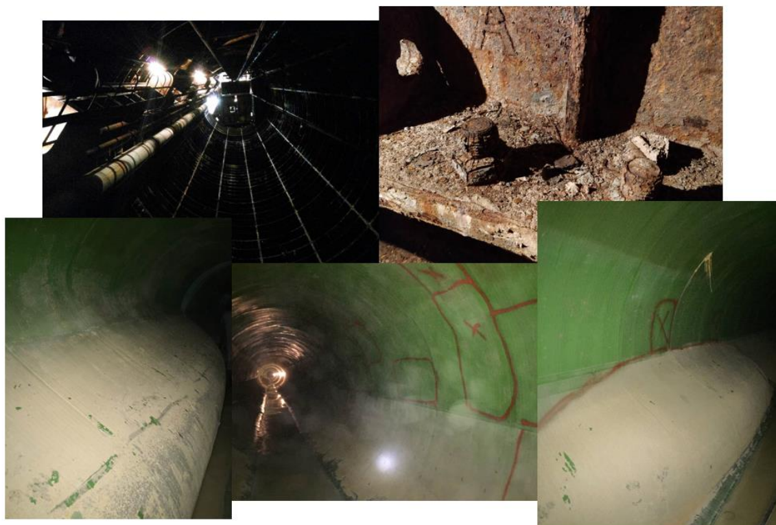
Figure 2. Defects noted during the inspection of the sewer in Kyiv*
